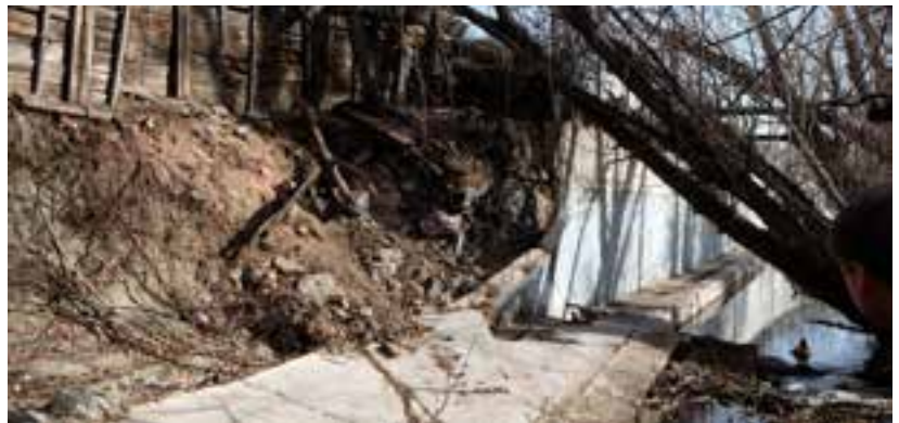
Failing retaining wall along Corridor pathway.
