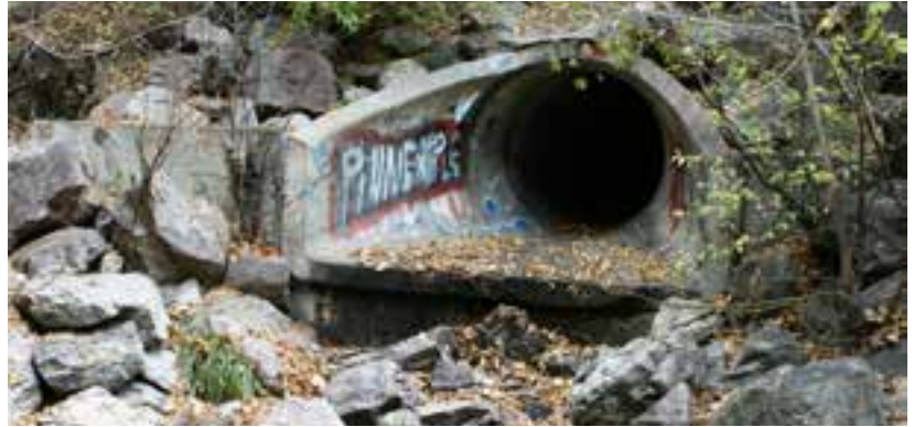
Erosion below a tributary drainage outlet along the channel.
