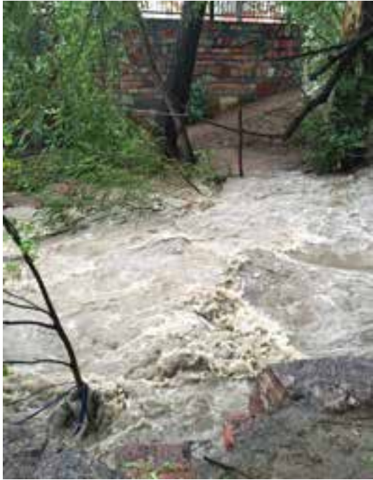
During periods of flooding, the channel water velocity creates localized flooding and increased channel erosion.
