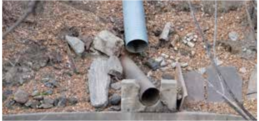
Disconnected or abandoned drainage pipe along the edge of the channel.
