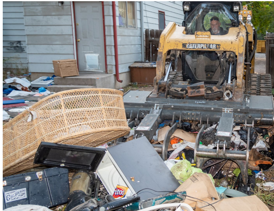
Code violation clean up
